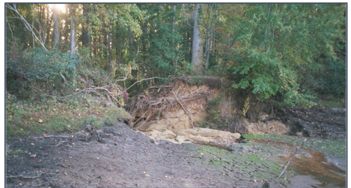
Tree roots growing into the dam's earth embankment causing failure.
